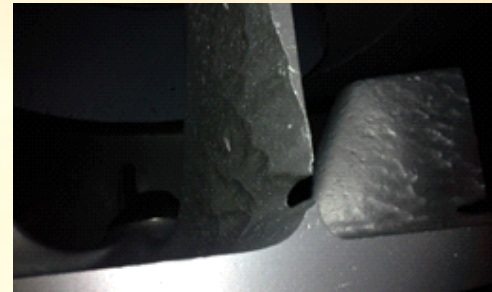
Figure 2 Damaged vanes of TV fan
